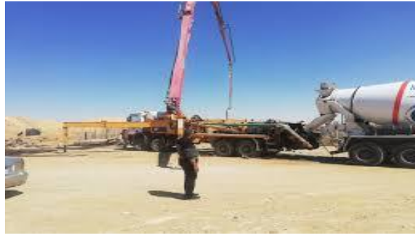
Figurer25 : Concrete Pump
